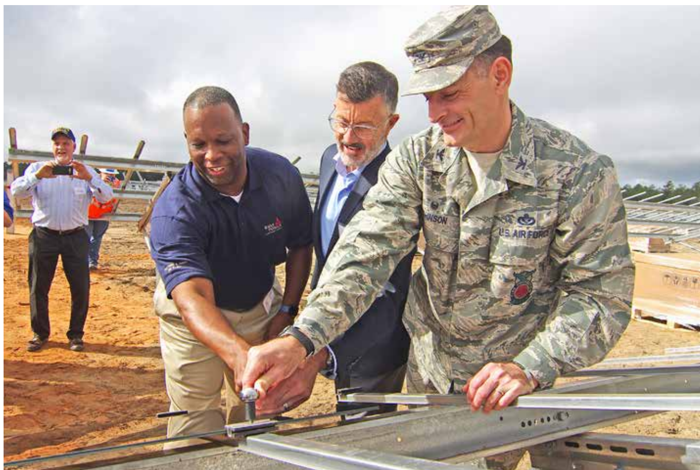
Mike Burroughs, Gulf Power; Ed Feo, Coronal Energy and Col. Craig Johnson, Eglin AFB, tighten the last bolt on the first solar panel at Eglin AFB.
